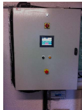
Main control command
