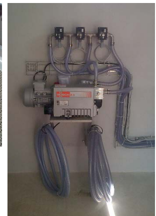
Equipment in the equipment room
